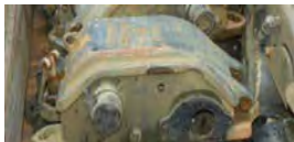
Switch Circuit Controller - Before
